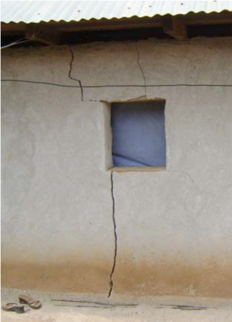
Figure 1a Vertical Wall Cracks in Adobe
