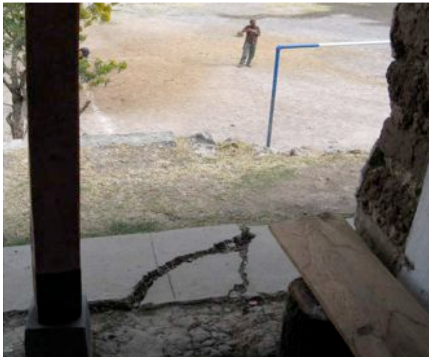
Figure 9b View From Building in Figure 9a (Fracture in foreground is same one shown in Figure 9a and it extends to person. Fracture difficult to see as it is partially filled with soil)
