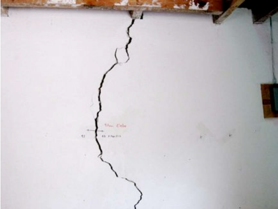
Figure 5e Type 5 Wall Crack Below Roof Beam
