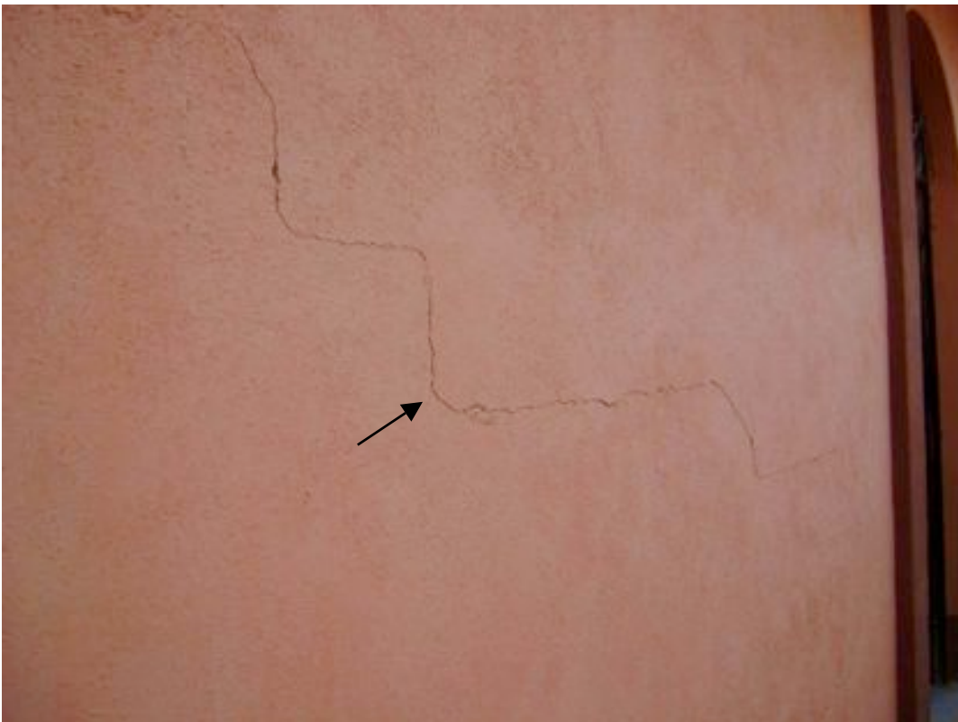
Figure 1d Crack in Concrete Block Grout
