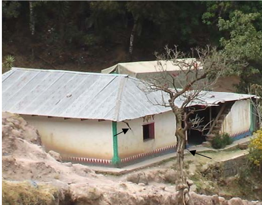
Figure 9a Damaged Building (note hole in wall, left arrow points to wall crack, right arrow points to fracture that extends into foreground)
