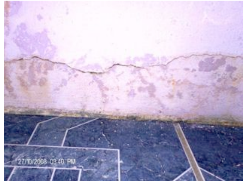
Figure 5d Type 4 Horizontal Crack
