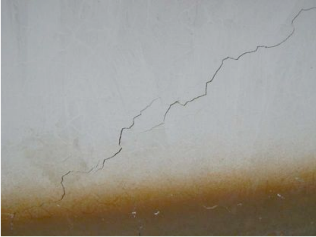
Figure 1c Incline Wall Crack in Adobe
