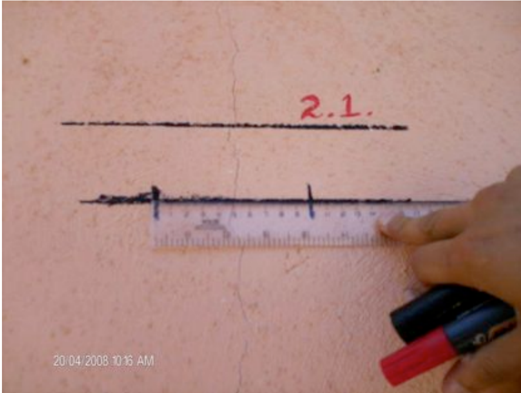
Figure 6a Measure Crack Width on Upper Line and Measure Width of Tick Marks on Lower Line
