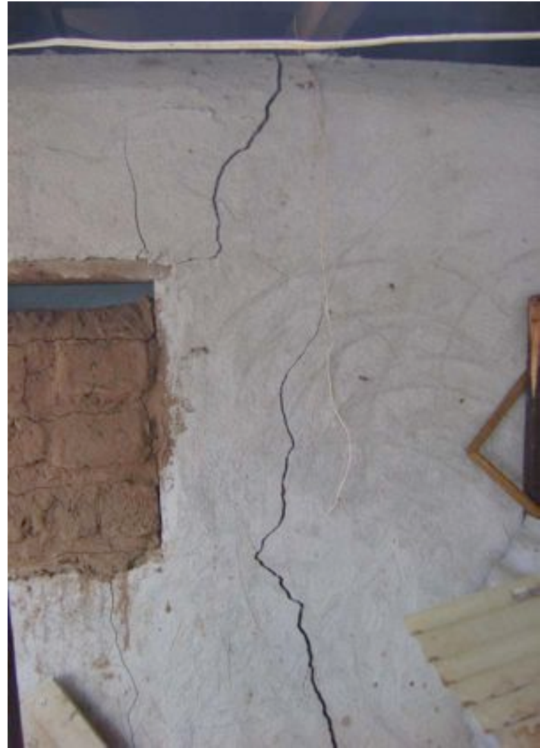
Figure 1b Vertical Wall Cracks in Adobe
