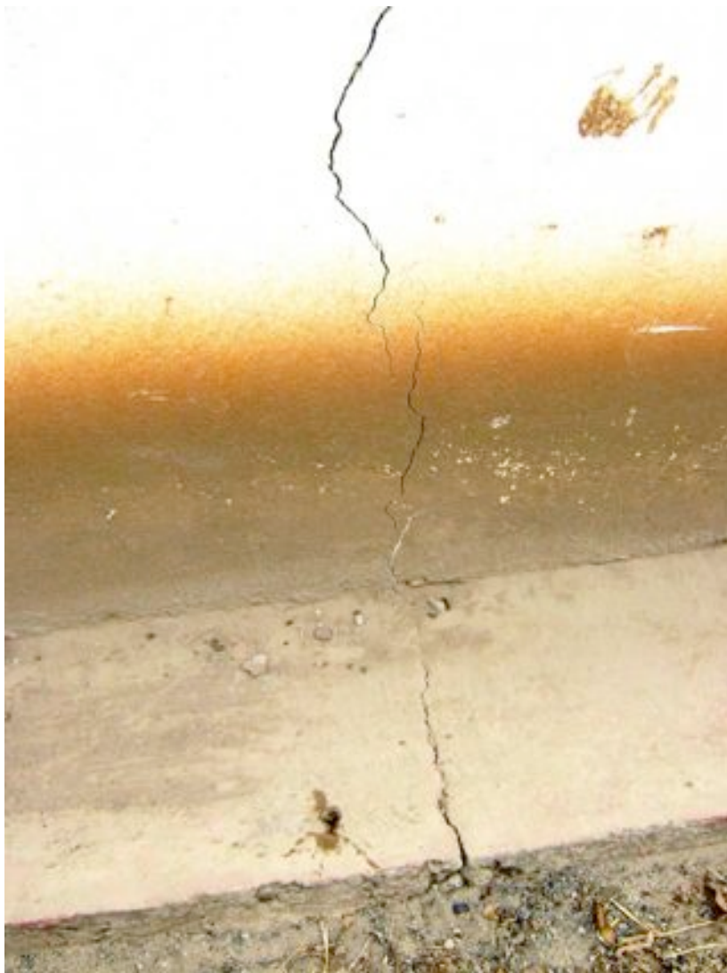
Figure 5c Type 3 Crack in Wall and Slab
